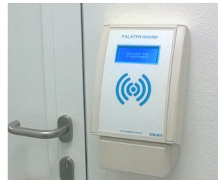
RFID access control readers
