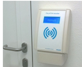
RFID access control readers
