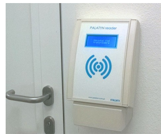
RFID access control readers
