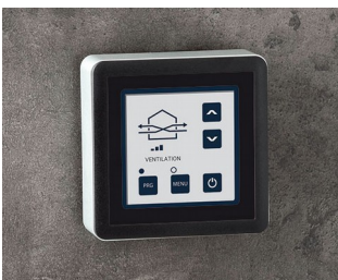
Ventilation system control
